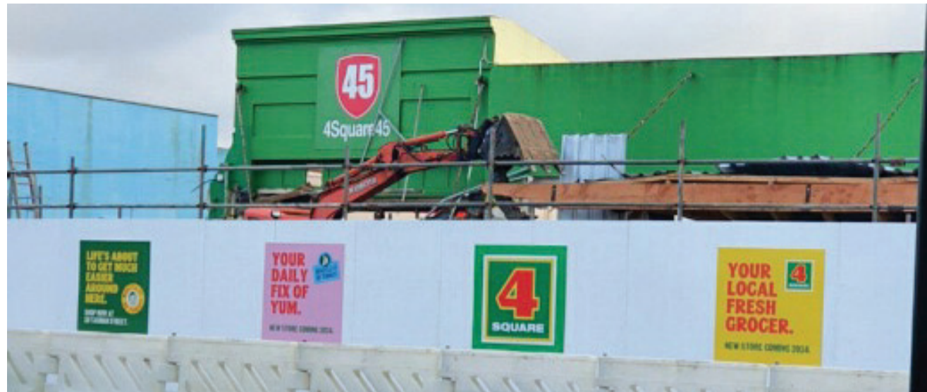
All that remains of the 4 Square 45 in Tasman Street, Opunake. The building is being demolished in preparation for the new store opening in 2024. By Wednesday morning, even this last part has gone.
